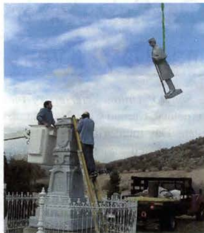
Crews await the top section to be moved into position for re-attachment to the main portion of the monument.
